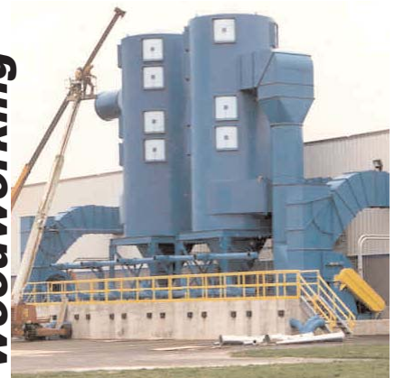
Here are two 544RF12 filters at a woodworking plant in Wisconsin.
